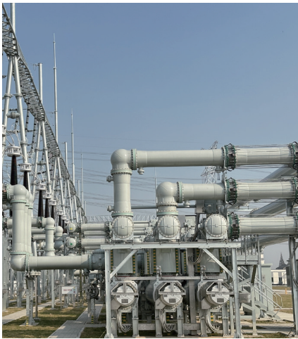
China | 363/550kV Substation
