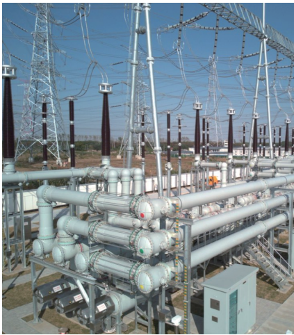
China | 363/550kV Substation
