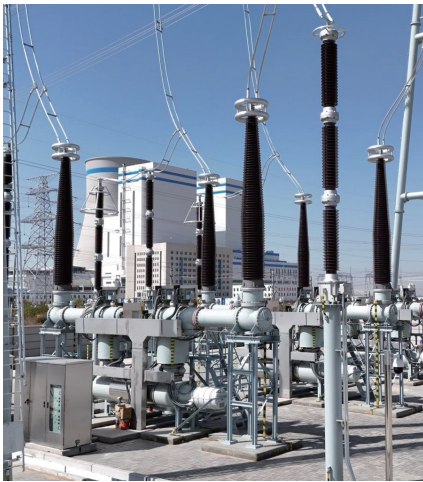
China | 363/550kV Substation
